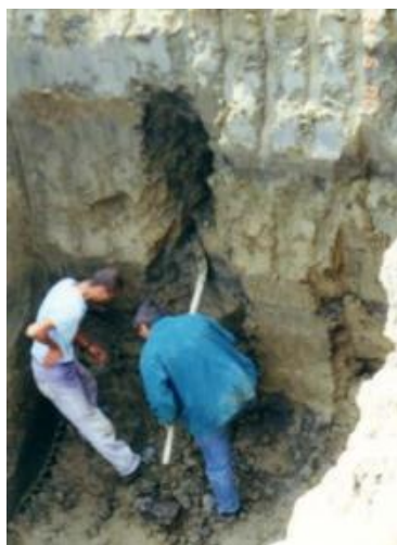
A piping's cavity level to the water side elevated. Tiszasas, no breach.
