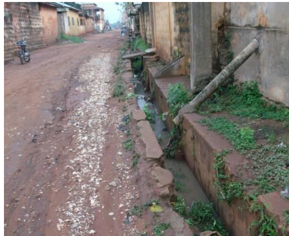
Photo 6: A section of rain water crest gate playing the part of waste water collector of a dwelling starting from a outfall in the district Tovè1 (district 3, Ouidah). Catch of sight Adoko E., June 2012
