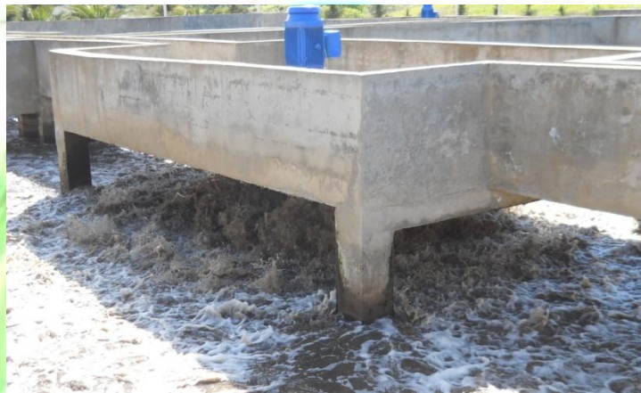
Figure 3: Biological Treatment, aeration basin
